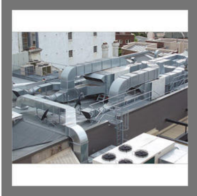
Commercial Air Conditioning Duct
