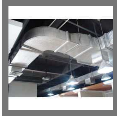
Industrial Air Conditioning Duct
